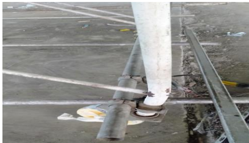
Picture 10 Damaged Mainframe Scaffolding Material
