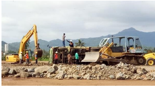
Picture 9 Overturned Dump Truck in Accessibility Zone
